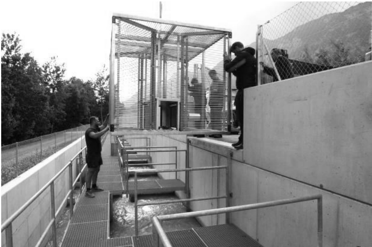
Fig. 3: Riverwatcher (with video tunnel) installation at hydro power station Langkampfen, installed in a guiding rack. The whole unit can be lifted for maintenance.
